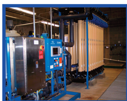
Coles Run Reservoir Filtration System
