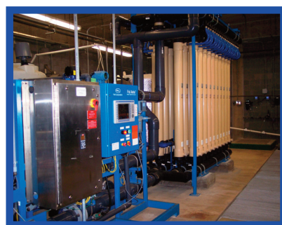
Coles Run Reservoir Filtration System
