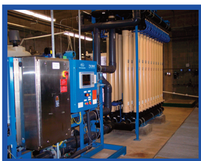
Coles Run Reservoir Filtration System
