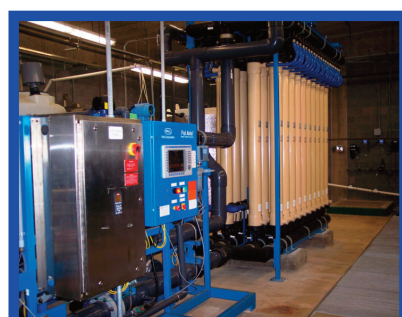
Coles Run Reservoir Filtration System
