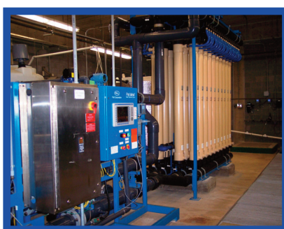
Coles Run Reservoir Filtration System
