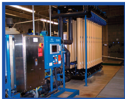
Coles Run Reservoir Filtration System
