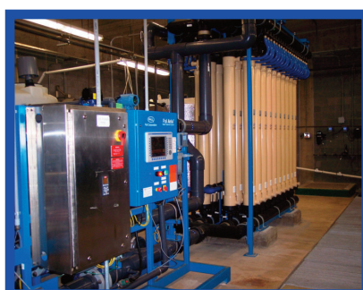
Coles Run Reservoir Filtration System
